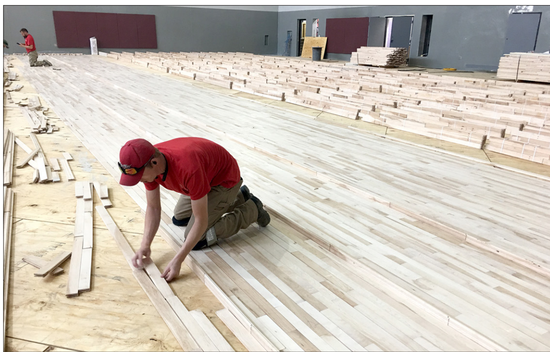
A worker is shown laying the floor inside the new gym at the high school in Grundy Center. (Courtesy photo)
